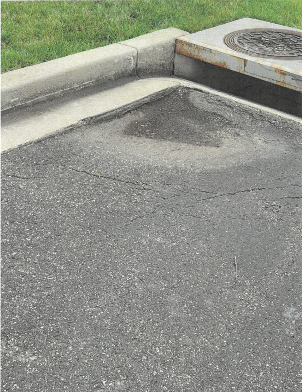
small pothole swim and tennis center parking lot
